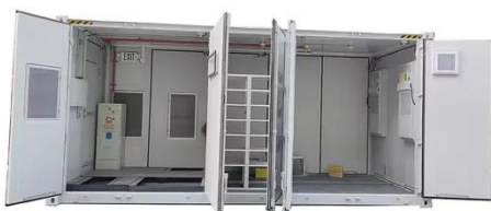
1075KW HH ESS
